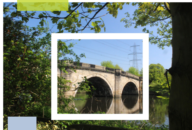
John Carr's Old toll bridge completed 1804 the Old Great North Road Ferrybridge Knottingley West Yorkshire Britain, UK.
